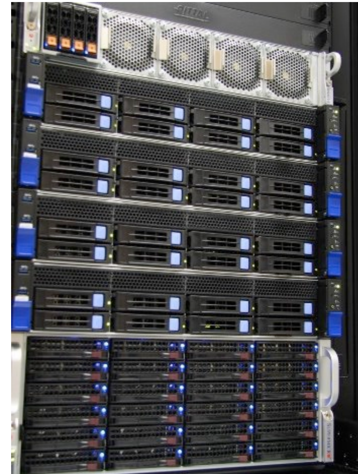
Installed nodes in HPC Room at Beutenberg
